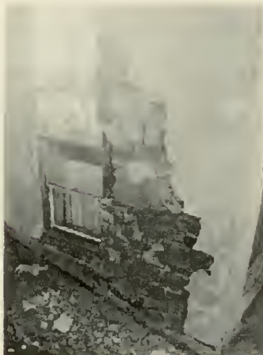
Figure 15. Location of second area of imminent wall collapse viewed from standing on the roof between the sanctuary and the hall
